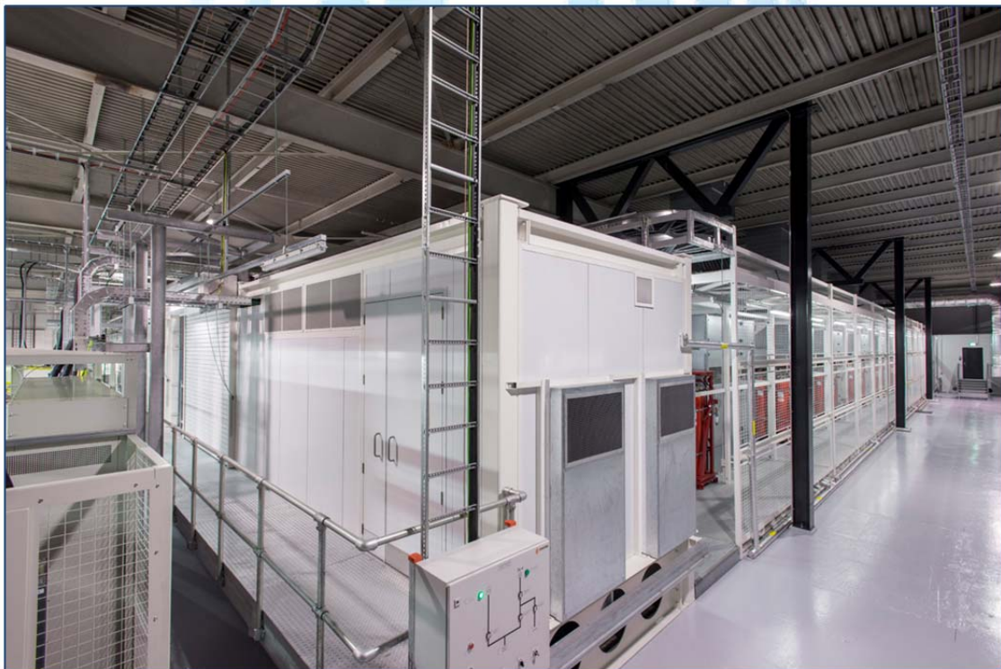
Verne Global's 100 percent, dual sourced renewable powered data centre campus in Iceland.
